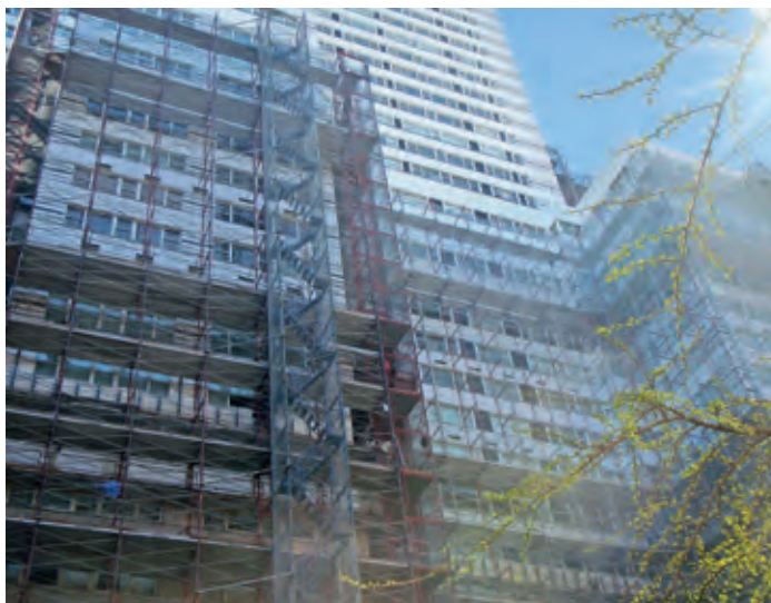
An ongoing building envelope renewal project is the renovation of the property on 215 East 68 th Street in New York City. The owner looked for a long-term façade repair solution which should also improve the energy efficiency of the building.
