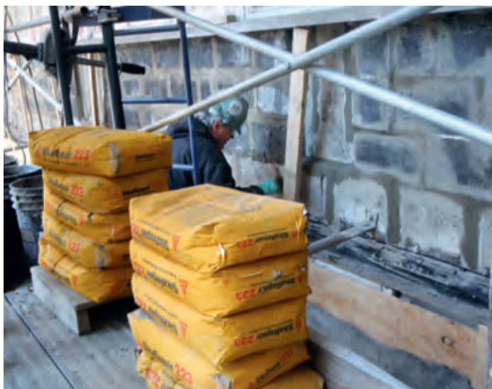
Repair mortar SikaRepair®-223 was selected to repair and patch the mortar joints, cracks and voids of the existing concrete wall structure to provide a uniform substrate before applying the membrane.
