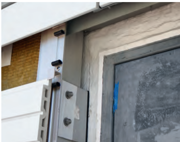
Sikagard®-560, a waterborne vapor permeable membrane was applied as a water and air barrier before installing the insulation and the new exterior rain screen cladding system.
