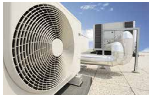
A/C units on a flat roof.
