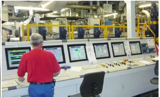
Central control desk of line 3
