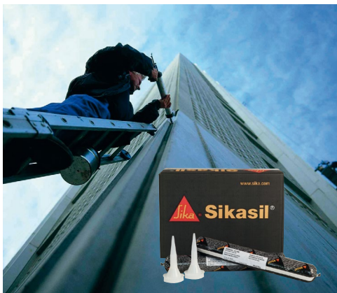
bottom: Gun application of 1-part sealants out of foil packs and cartridges (on-site application)
